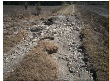
Access roads impassable.
