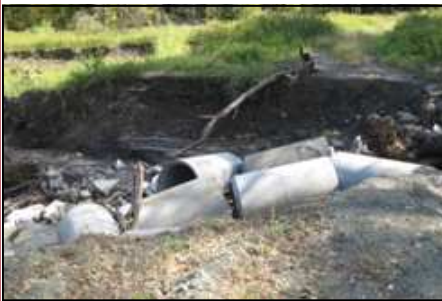
This culvert crossing was destroyed in the heavy September rains. The force of the water and the large debris caused two 42" concrete culverts to be blown out of the crossing with ease.
