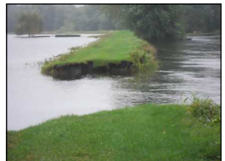
Large section of dike blown out.
