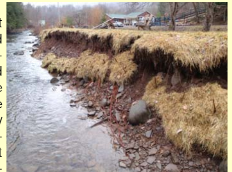
Eroded streambank with inadequate buffer.
