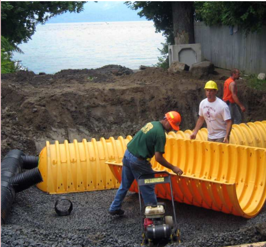
Crews from the Warren County Soil and Water Conservation District and the Town of Bolton Highway Department install stormwater infiltration chambers designed to reduce erosion and flooding while preventing pollution from entering Lake George.
