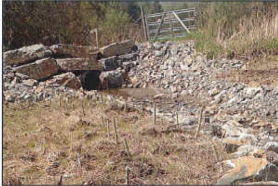
AEM Tier 4 Access Road and Culvert Crossing Project completed October 2015 – with willow plantings for channel stabilization in April of 2016
