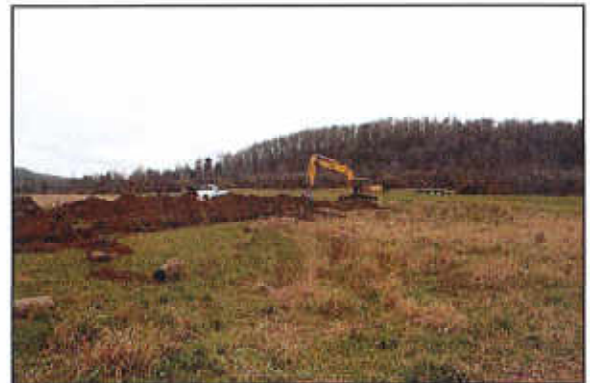
WASCOB outlet repair in November 2016 which included resizing the pipe and re-grading the spillway.
