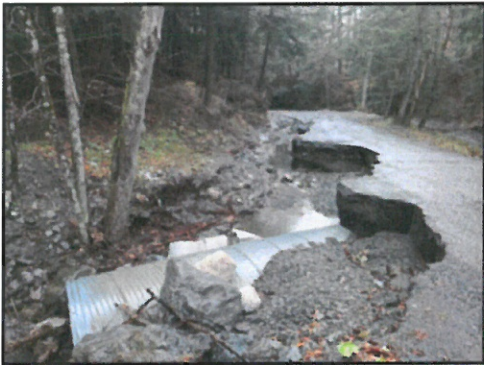
Undersized culvert post storm
