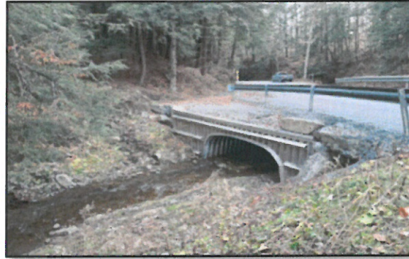
Newly installed arch culvert sized to handle a 500 yr storm
