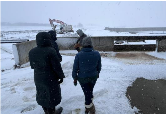
A project in the final stages of completion for a waste storage and transfer project in the Town of Covington.
